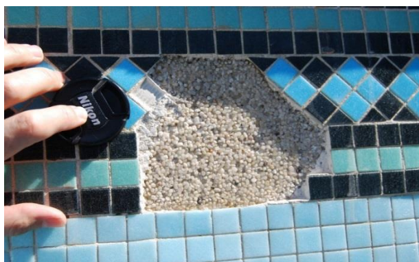
An example of a pool shell where tiles were applied over 'Pebblecrete' with generally poor adhesion of the tile adhesive.
