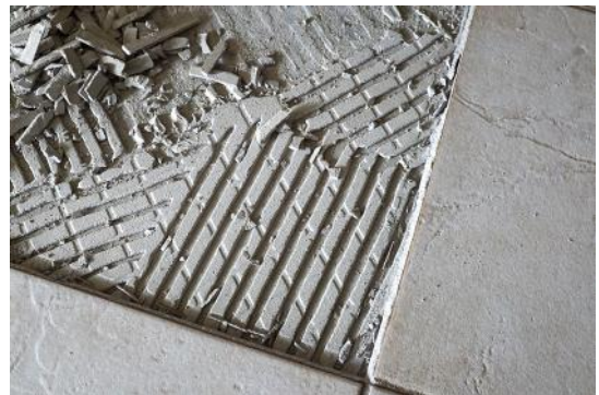
An example of a tile that was drummy and had bowed slightly off the adhesive bed (it had to be re-stuck).
