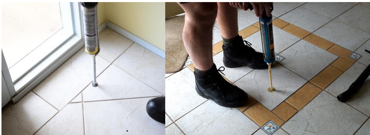
Injecting ARDEX RA56 at left and Dunlop Ardit Crack Filler at right
